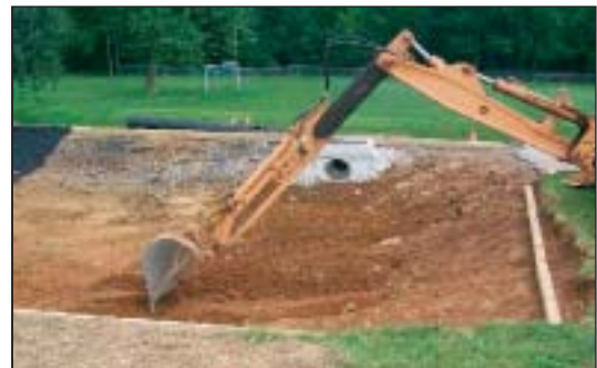
1. The subsurface infiltration bed located beneath the porous pavement must be excavated without heavy equipment compacting the bed bottom. (Cabill Associates Photo)
