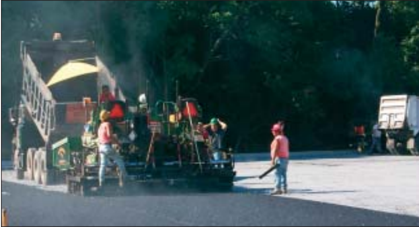
4. Clean (washing) uniform graded aggregate is placed in the bed as the storage medium. (Cabill Associates Photo)
