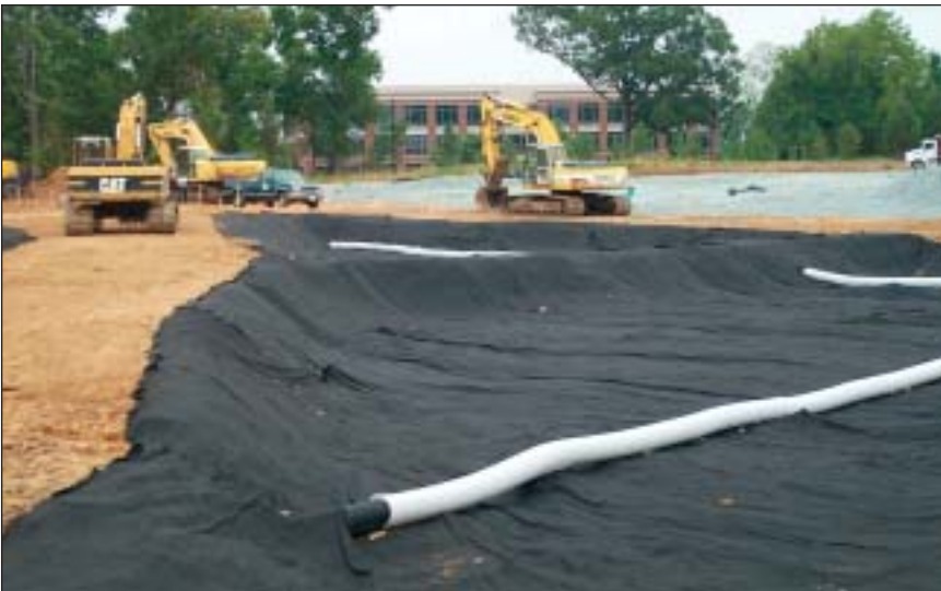
5. The asphalt is laid down just like conventional asphalt. (Cabill Associates Photo)
